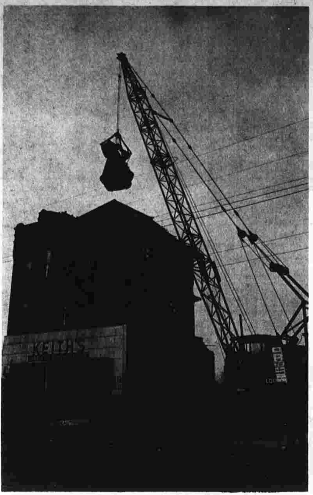
Tower Cone, Not a Space Capsule The 1800 Keith Building on N. Main St. went "the way of old bricks" today, to make room for North End Renewal. The tower cone being removed, and one other already down, have been spoken for. The Ever Ready Destruction Co. of Newton, which is demolishing North End properties, has a customer for the two cones. The three-story-plus-attic Keith Building, one of the tallest in Manchester, is one of the last structures in the development area to come down. Still awaiting destruction is the building at Depot St., Edward Rybeck, executive director of the Manchester Redevelopment Agency, has predicted North End Renewal completion by next October or November. (Herald photo by Fintz.)
